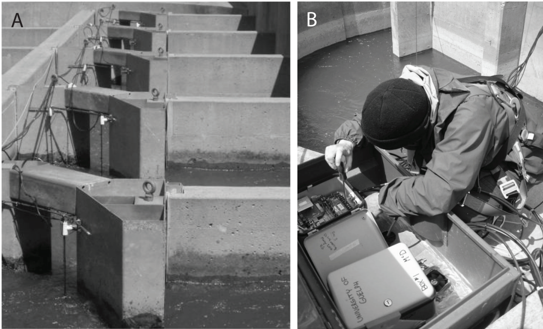
Figure 18.3 (A) Passive integrated transponder (PIT) tag array installed in a vertical slot fish-way. The antenna wires encircle each of the vertical slots and connect to (B) an antenna multiplexer, logger, and power supply in a secure and weatherproof box (photo [A] by J. Thiem, Carleton University, with permission; photo [B] by S. Cooke).
